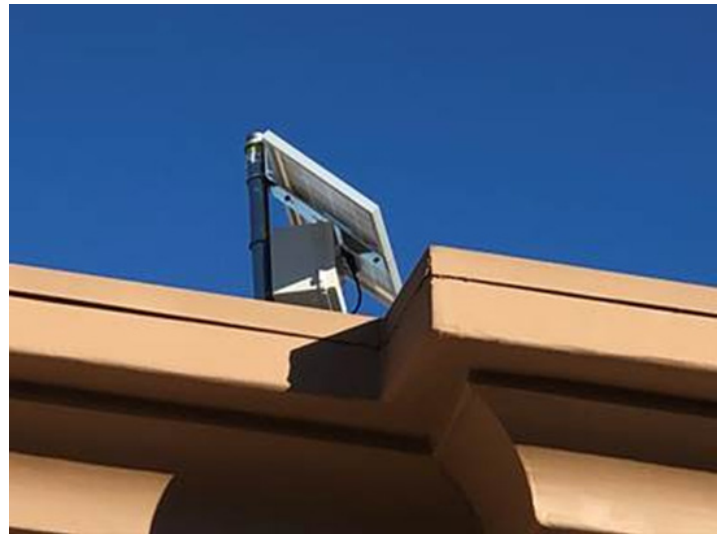
Finished Repeater, Ground View:
